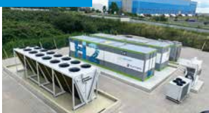
2 MW Electrolyzer with swap storage filling
